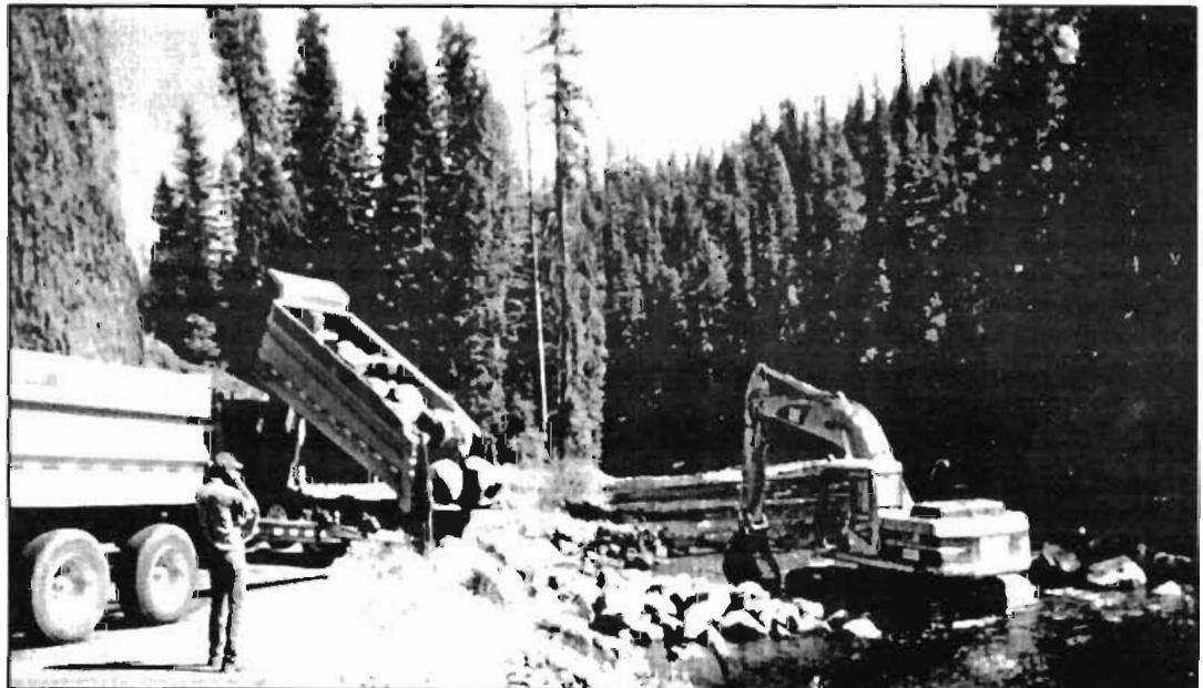
Unloading huge rocks to be used for barb deflectors and placed huge boulder clusters like those placed directly behind the excavator.
